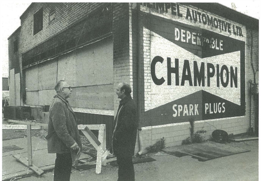
Both Heimpels survey the charred front entrance of their building. Fire occurred in the early morning hours of April 15. Unless everything is clearly spelled out, and fully understood, in an insurance policy, compensation for damages can be time consuming and frustrating, Heimpel said.
